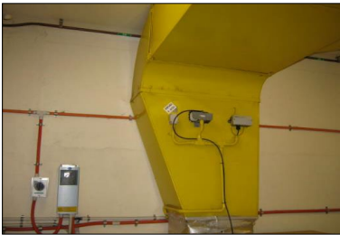
8724: B Block, A/C Heater Bank
