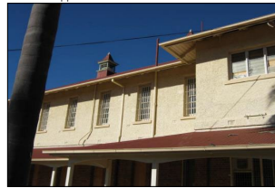
X Block: Vent pipes
