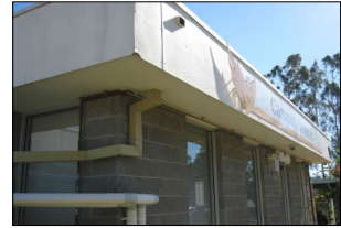
8764A / 8765A: V1 Block, fascia & eave soffits
