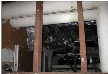
8729 A: B Block, Debris in ceiling space, on timber studs
