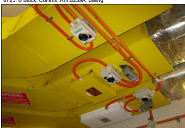
8726: B Block, A/C Heater Bank
