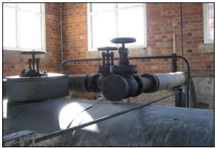
Boiler: Q Block, flange gaskets
