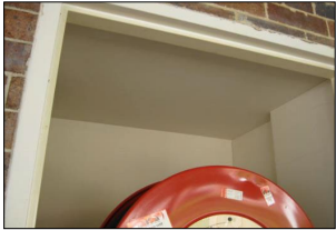
8754: R Block, Fire Hose Reel Cabinet, ceiling
