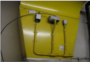
8727: B Block, A/C Heater Bank
