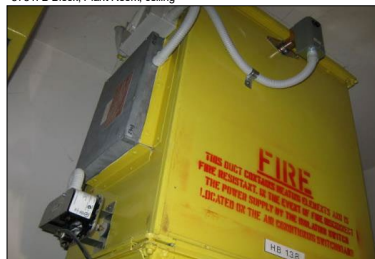
8732: B Block, A/C Heater Bank
