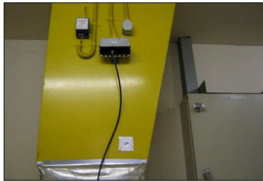
8728: B Block, A/C Heater Bank
