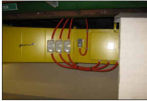
8758: O Block, A/C Heater Bank
