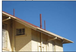
X Block: Vent pipes
