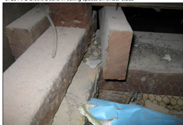
8729 B: B Block, Debris in ceiling space
