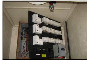
W Block: East Switchboard, backing board & lining board
