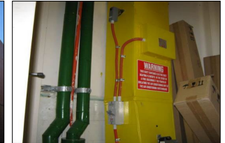
8759: P Block, P102, A/C Heater Bank
