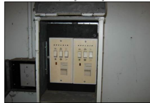
W Block: West Switchboard, backing board
