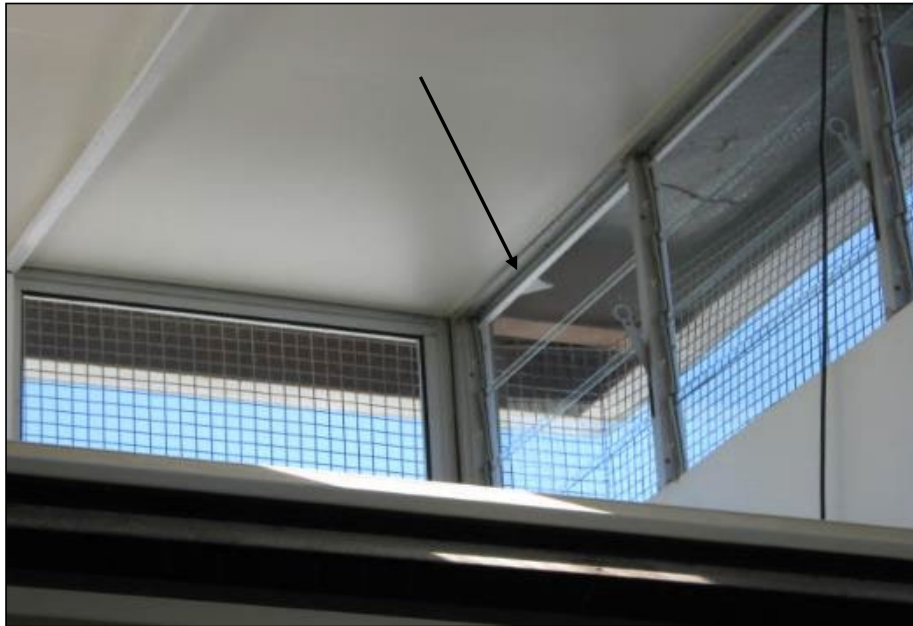
V1 Block: Skylight Debris
