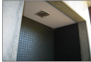
8763 A: U Block, ceiling throughout
