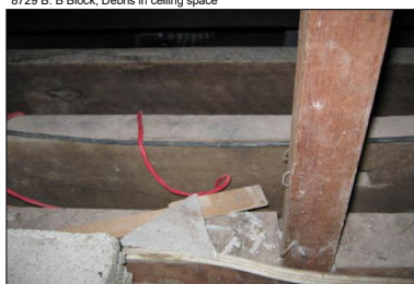
8729 C: B Block, Debris in ceiling space
