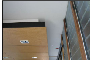
8763 B: U Block, ceiling throughout
